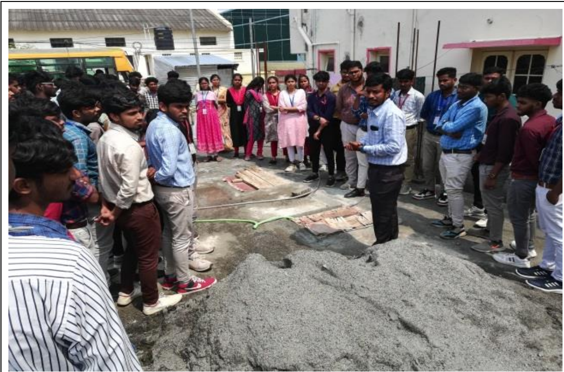
Fig.9: Third year civil engineering students visited an ongoing construction site located at peelamedu, Coimbatore which is constructed by JAS associates.
